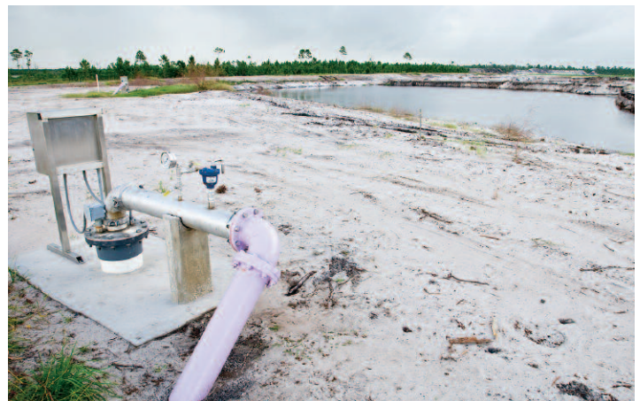
At a new treatment facility, purple pipes indicate this is a reclaimed water system.
